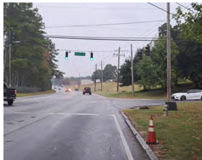
Signalized Intersection at Marbut Rd has Curb Damage and No Marked Crosswalk, Pedestrian Signals, or Sidewalk
